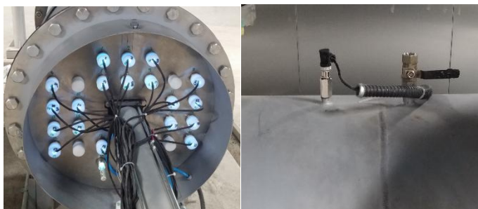
Water treatment systems operating examples
